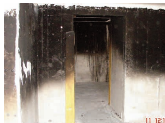
Figure C-7: Interior View of Burn Prop
